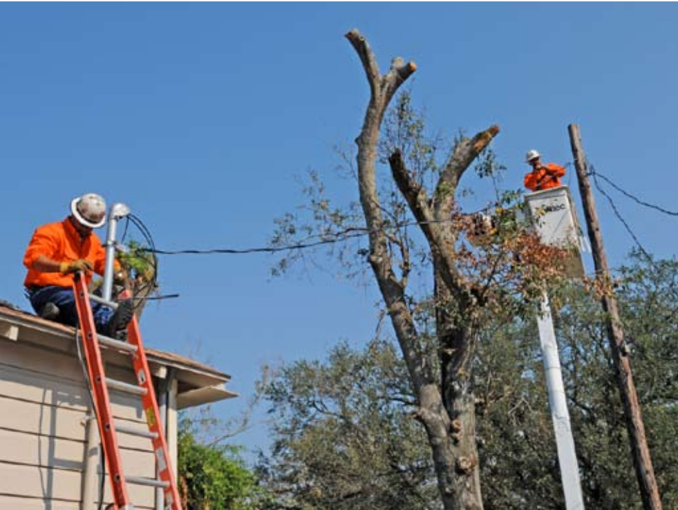
Line mechanics repair a service drop, bringing yet another customer back online.
